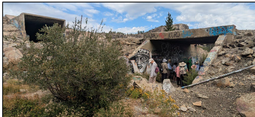
Our group explores the 1912 underpass for California State Highway 37. The east portal of Tunnel 7 is in the upper left. Photo by Steve Edelman
